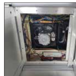
A5. Condenser compartment
