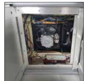
A5. Condenser compartment
